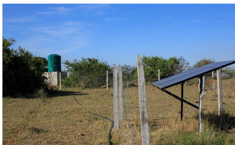
Figure 3. Solar system installed during Shewula wetland restoration project with support from the EEF
