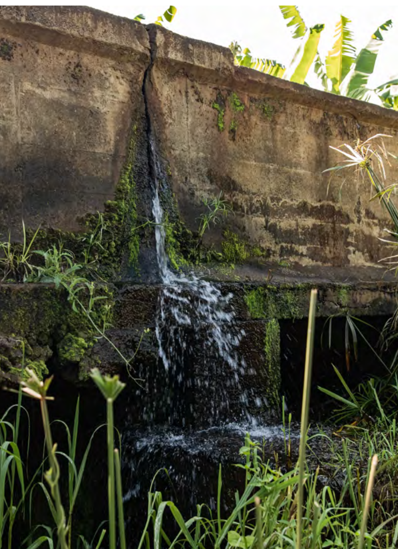
▲ A cracked canal wall as a result of high water pressure flowing during heavy rain. (Charity Kishoyian)
