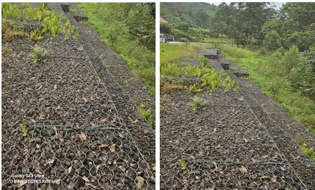
Figure 11. Examples of gabions along the Kigali-Rulindo-Gakenke and Musanze roads
