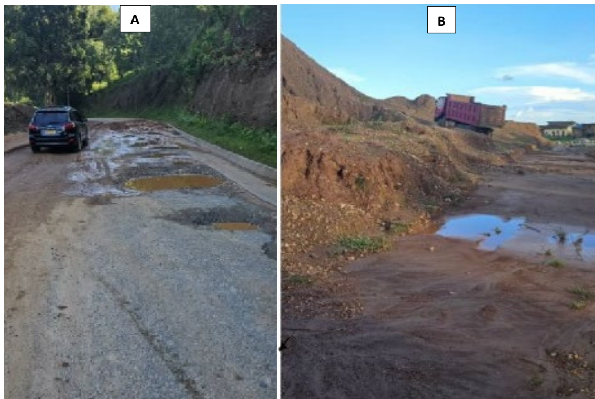
Figure 5. Damaged roads (A) and quarries (B) along the Muhanga, Ngororero, and Karongi route
